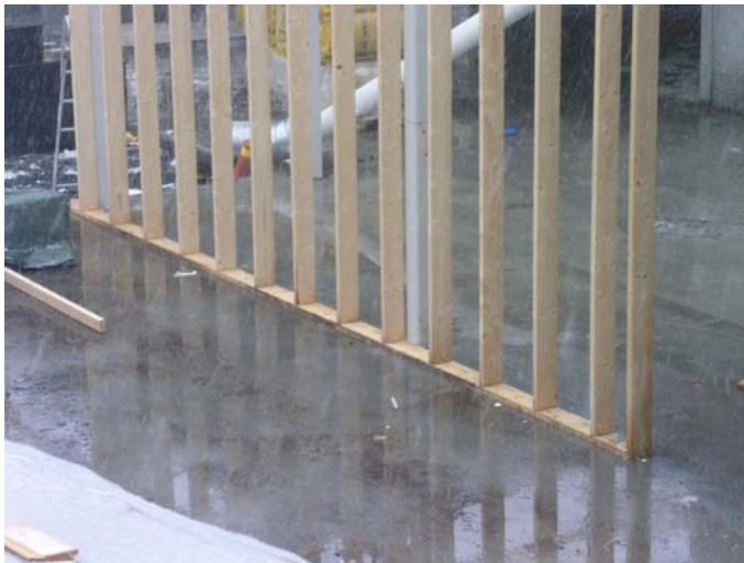
Figure 7.1 Framed wall unprotected from rain and melting snow and with visible signs of soaked up water.
